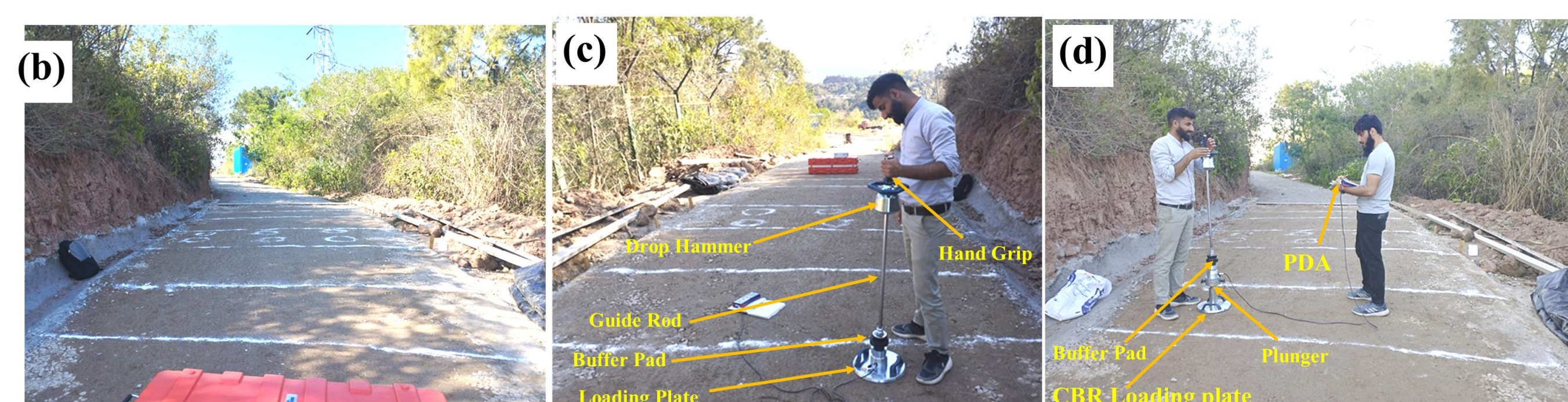
LWD and Field CBR tests on field: (a) Compaction of base layer, (b) Marking of exact test locations, (c) LWD Testing, (d) Field CBR testing
